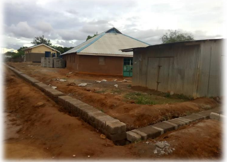
Akatgol Presbyterian Church in Juba stepped out on faith and started a school. SSEPP funded the construction of two classrooms. The school community recently advocated for and received government funds for a much-needed security fence. Praise God for the good collaboration!
